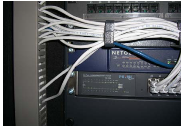
Pic 9 Side cable management and cable entry 300mm cable tray shown
