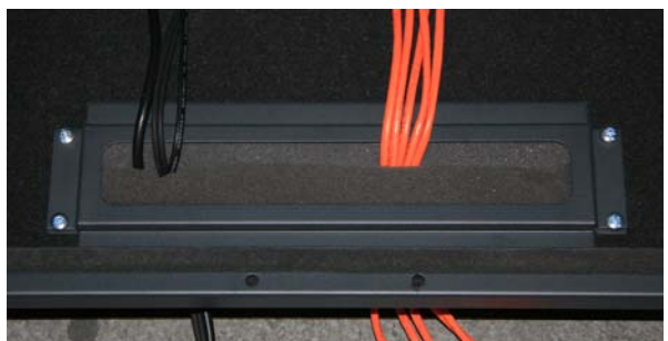
Pic 5 Cable entry box fitted to base of cabinet
